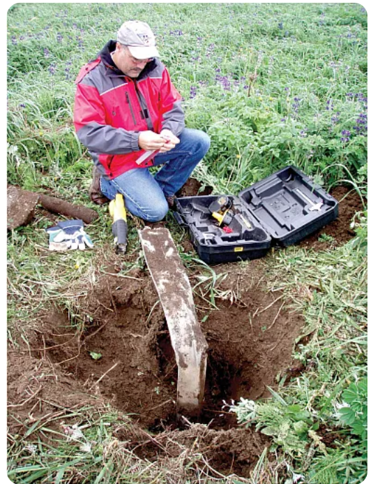
A groundwater monitoring well being decommissioned by NOAA personnel. Photo courtesy of Greg Gervais, NOAA Pribilof Project Office.
