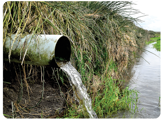
Water flows out of a tile drain into a nearby ditch. Photo by Jane Frankenberger.
