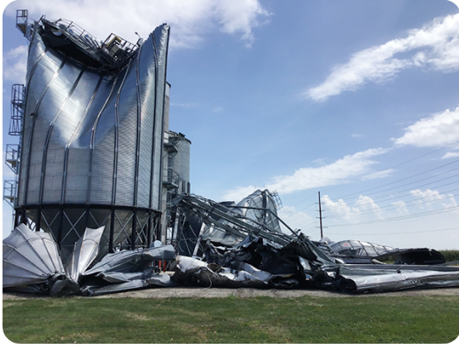
Grain bin damaged by August derecho in Iowa. Source: weather.gov .
