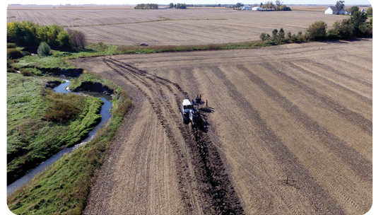
Prep begins for installation of a saturated riparian buffer in Story County, Iowa. Photo by Lynn Betts, USDA-NRCS.
